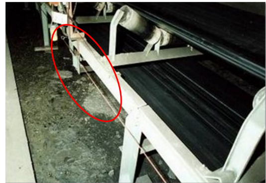
Fig.3. The deployment of fiber optics for DTS.
