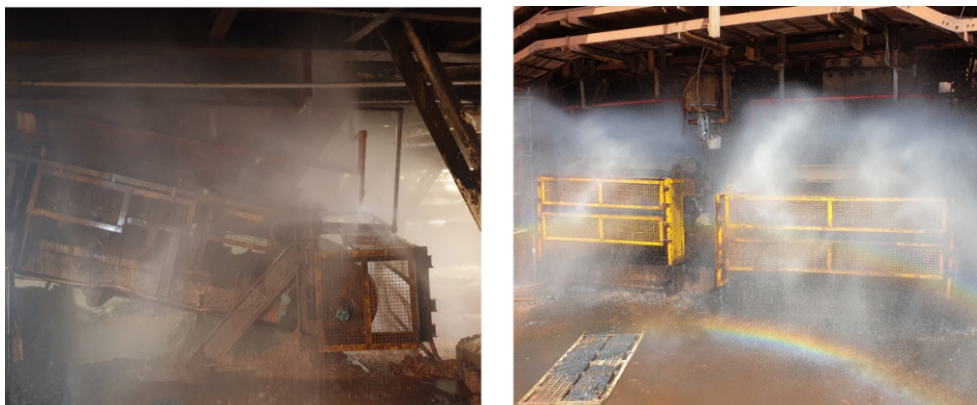
Fig.17. The activation of water suppression system.
